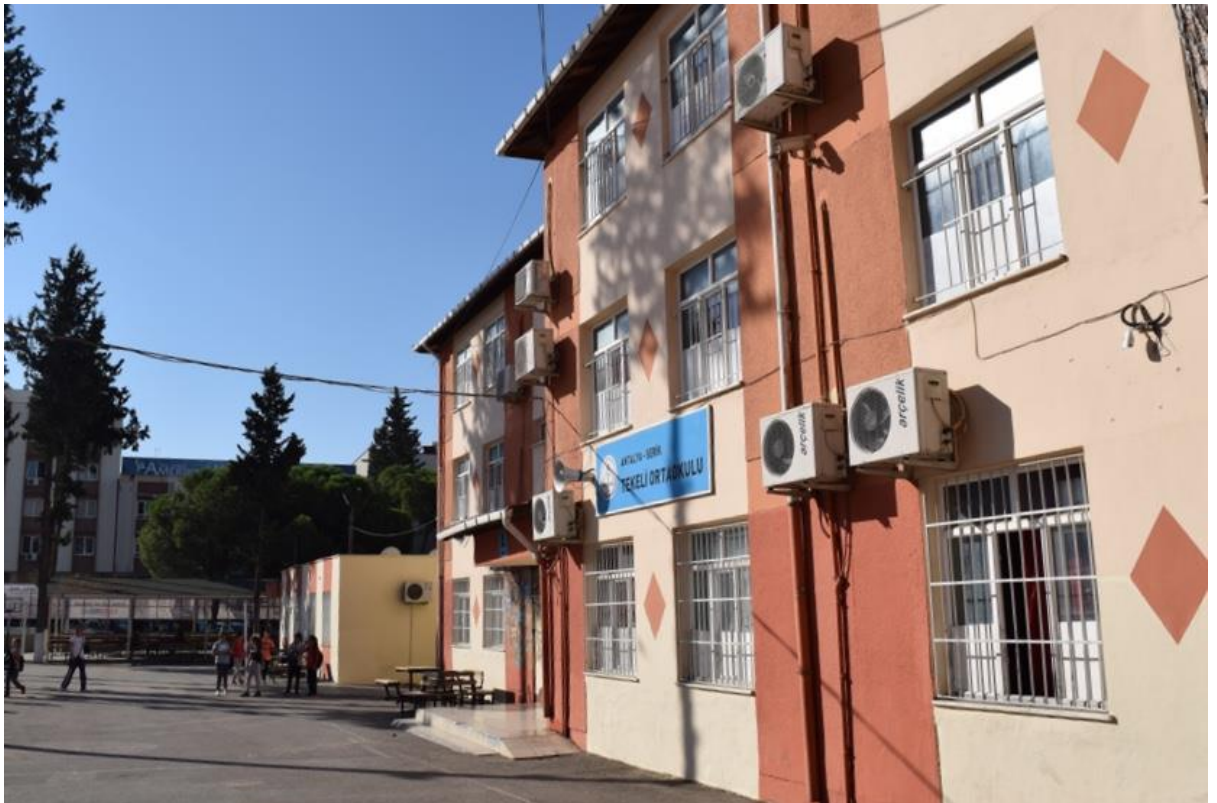
Figure 3.4 Air conditioners used for heating and cooling
