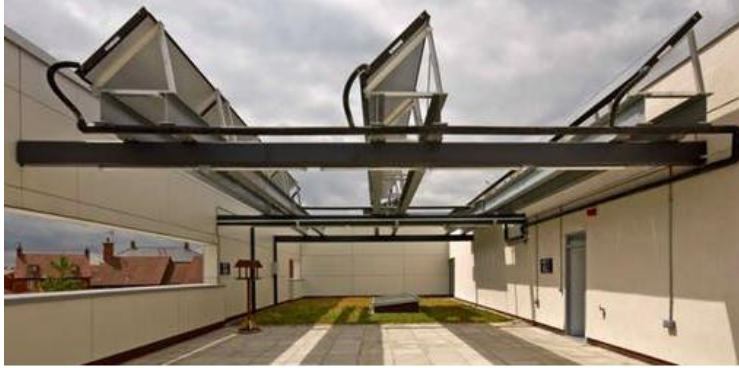
Figure A9 Solar panels in the school (Bonehill, 2016).
