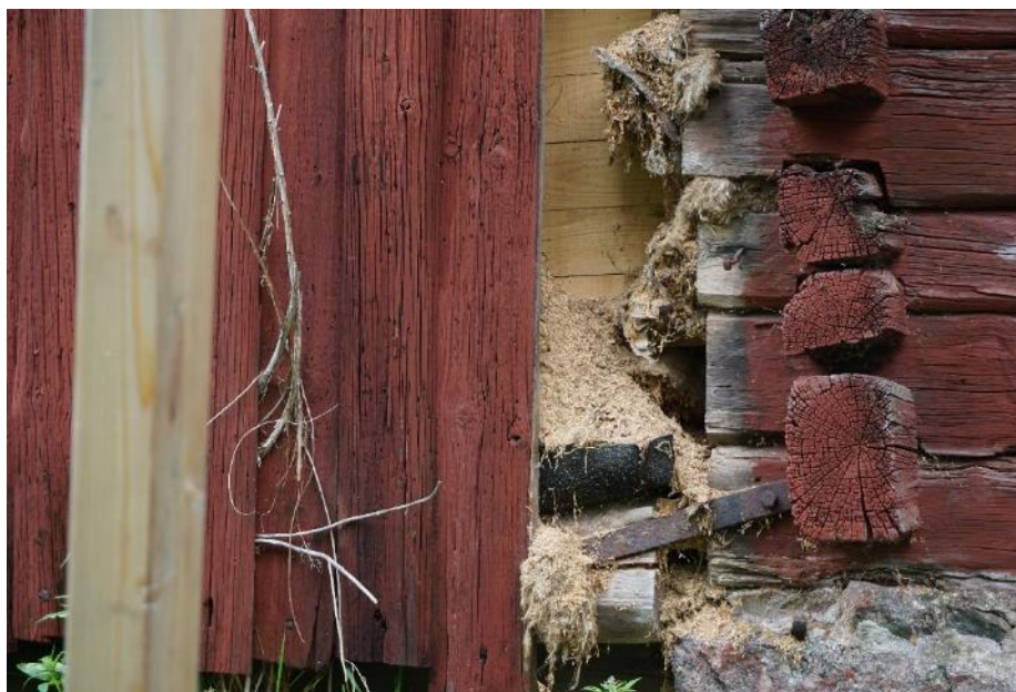
Figure 23: A detail of the damaged, termite-eaten wooden wall of the Red House. Photography by author. 9 July 2016.
