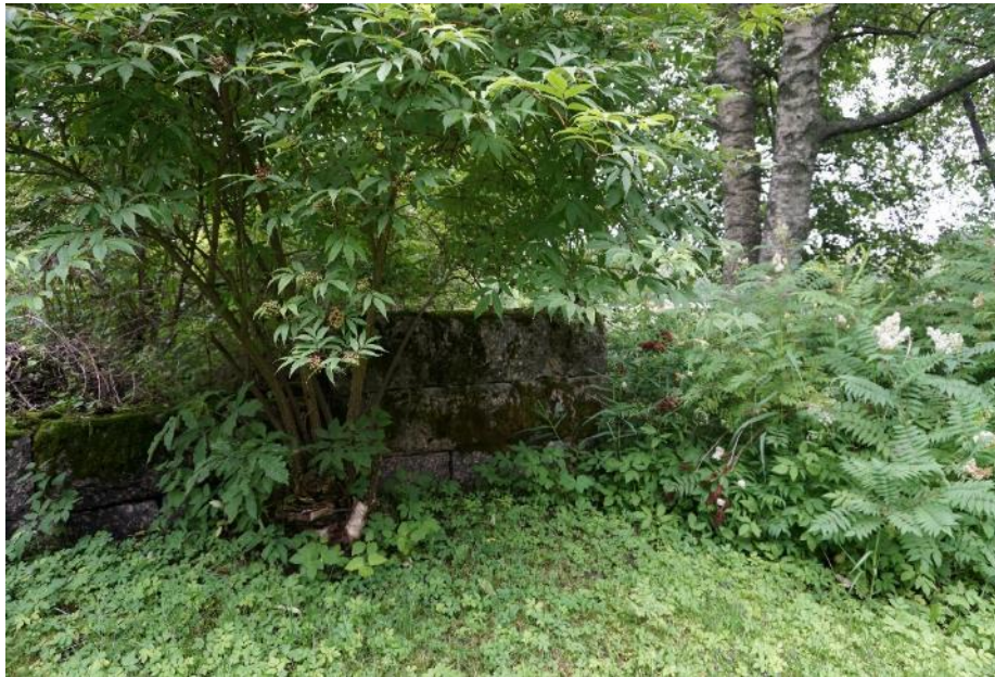
Figure 21 A photograph of the foundation stones of the beam house covered in moss and lichen by the Lake Vuorijärvi. Photography by author. 9 July 2016.
