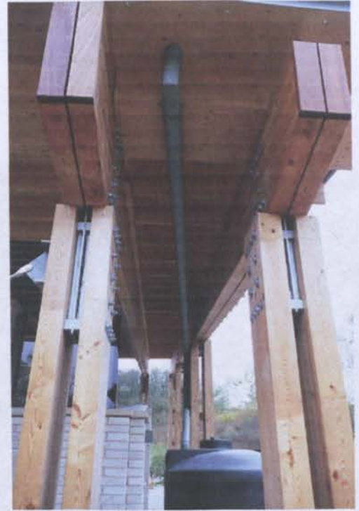
Figure 5.35 Visible rainwater harvesting system Source: Author
