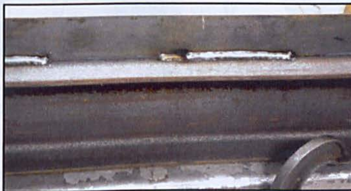
Figure 4.5: Connection of fish plate to boundary members using intermittent fillet welding on both sides of fish plate
