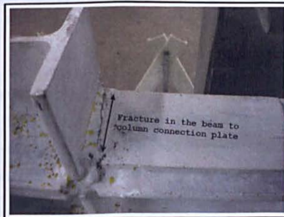
Figure 5.8: Fracture in weld of beam to column connection plate during the last cycle of testing for frame-only specimen
