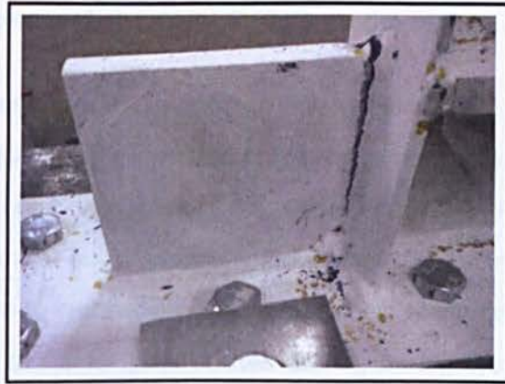
Figure 5.58: Weld fracture between stiffeners and column connections
