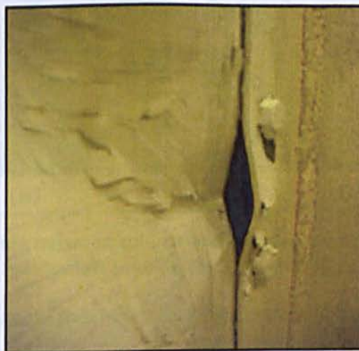
Figure 6.3: Occurrence of local buckling in the steel plate and fish plate
