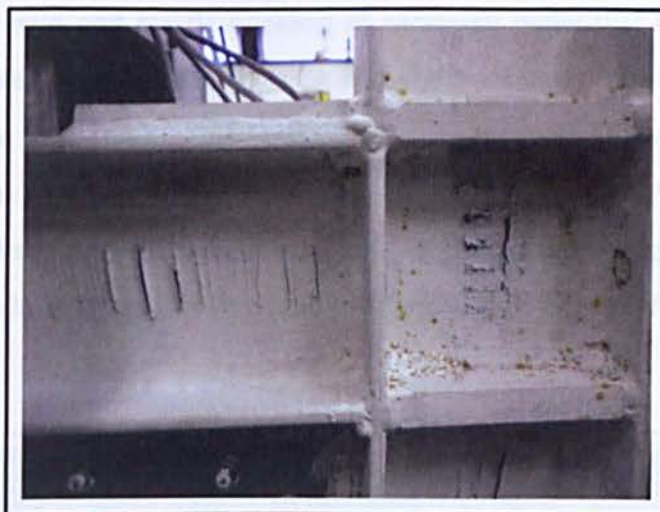
Figure 5.49: Formation of plastic hinges at the end of beam
