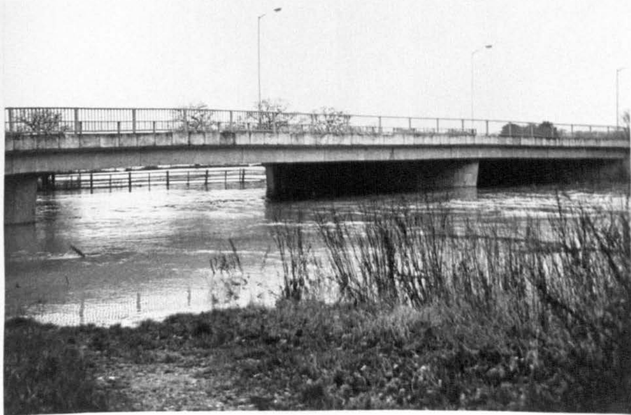
Plate 34. High Flow through Downside Bridge - Event 32.
