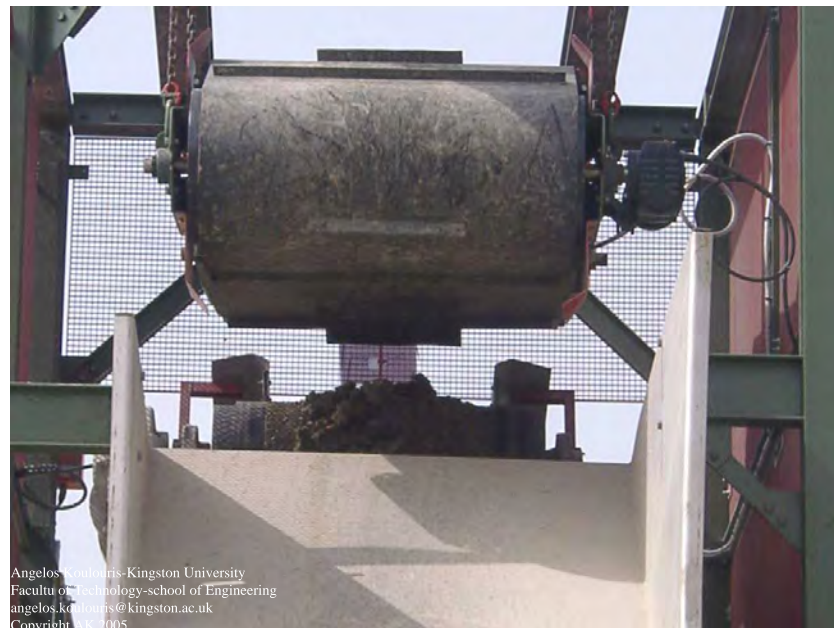
Figure 5.3: Electromagnet located after the primary jaw crusher used for removal of reinforcement.
